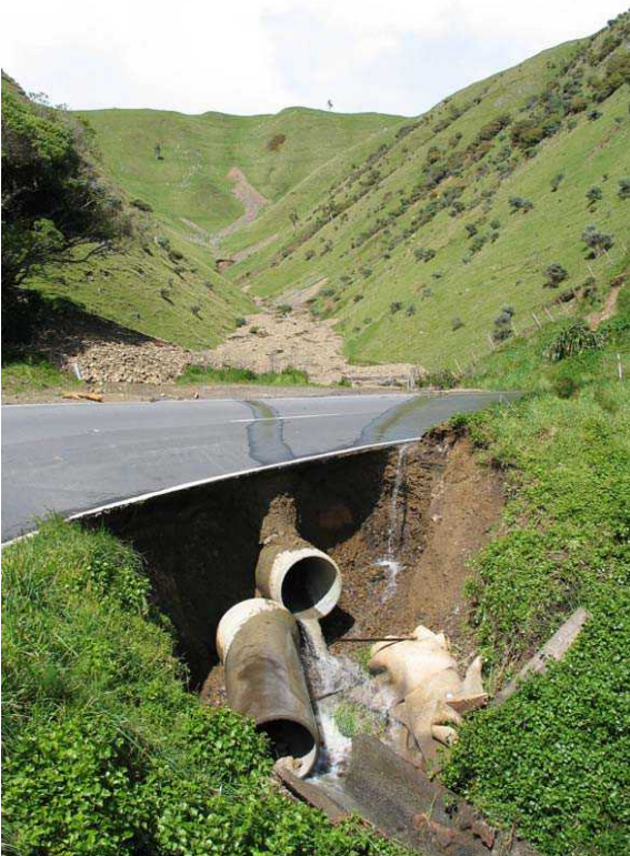
Council's Paekākāriki Hill Rd was severely impacted
