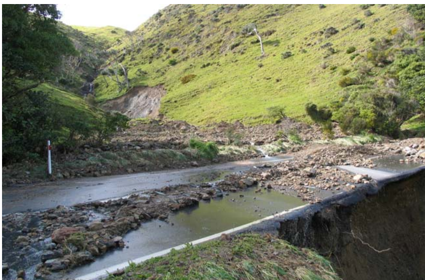
Figure 12. Ground view of damage Site 4 on the lower Paekakariki Hill Road, showing the soil slump and gravel debris deposited in the gully just above the road, where it has been trapped behind a farm fence. Some gravel was also washed across and down the road. Fill collapse has undermined the road edge here over a distance of about 10 m (the area in shadow bottom right).
