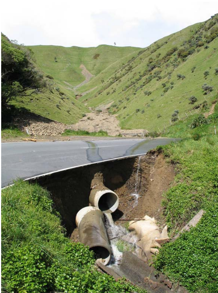
Figure 14. Damage Site 7 on the Paekakariki Hill Road (Site 6 is a debris lobe from the steep gully out of picture to the left – see Figure 16). At this site a large volume of gravel has been carried down from the head of the Hill Road Gully as a debris flood. However, here all of the gravel was trapped behind the fence and gate above the road (see Figure 15 also). Only flood water appears to have crossed the road at this location, washing out the road edge fill and undermining the road. No gravel debris has been carried across the road. The low volume of water flowing from the broken culvert pipe here is seeping through the gravel, which has completely blocked the culvert intake above the road.
