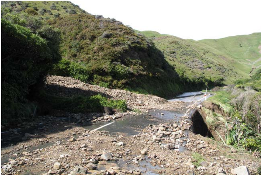
Figure 13. Damage Site 5 on the lower Paekakariki Hill road (see Figure 2), showing debris flood gravel from a small gully spilled across and down the road. The road edge fill has also collapsed and undermined the road.
