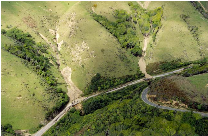
Figure 11. Aerial view of Sites 4 (left) and Site 5 (right) on the Paekakariki Hill Road (see Figure 2) showing the slips, gully erosion, and debris flood gravel deposits across the road, and undermining of the road due to fill wash-outs and collapses.
